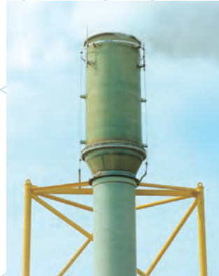
Chimney swirl droplet separator at BASF
