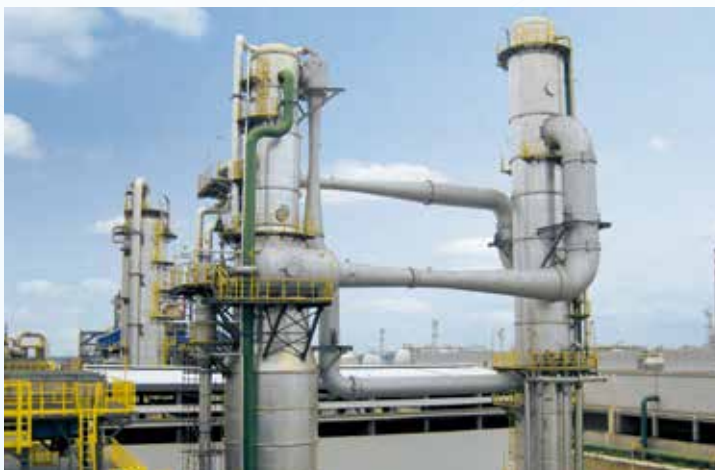
24 MW steam jet chilling plant Petro China/Sichuan refinery, cooling of 2 300 m 3 /h from 29 °C to 20 °C
