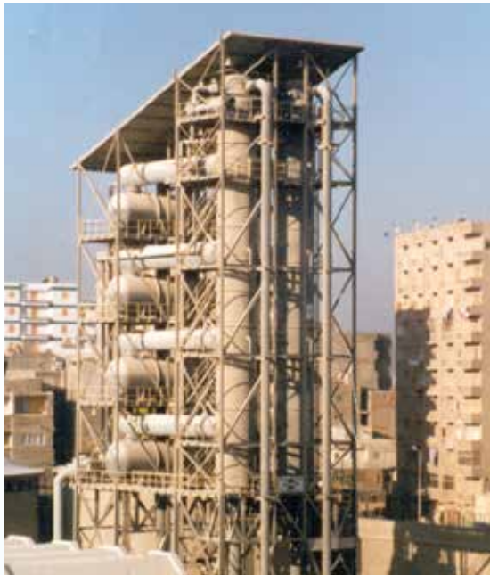
28 MW steam jet chilling plant in Egypt, cooling of 1 600 m 3 /h from 35 °C to 20 °C
