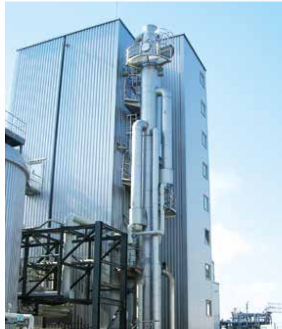
About 1.4 MW steam jet chilling plant in Stendal, cooling of about 72 m 3 /h from 25 °C to 8 °C
