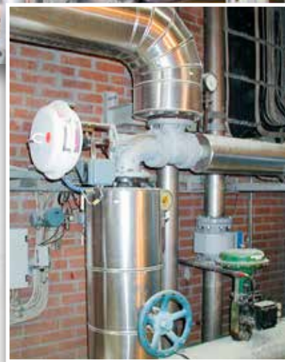
Körting thermocompressor in a paper factory
