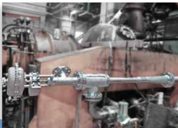
Körting thermocompressor installed at a paper machine
