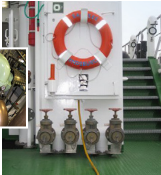
The suction hosepipes can be connected to these four connections.
