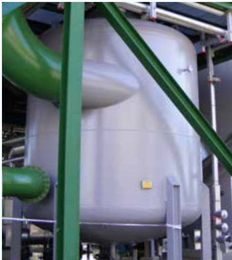
The buffer/separator tank discharges fatty components at the overflow.
