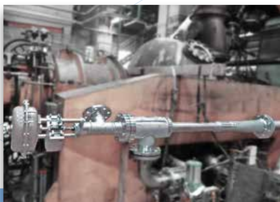
Körting thermocompressor installed at a paper machine
