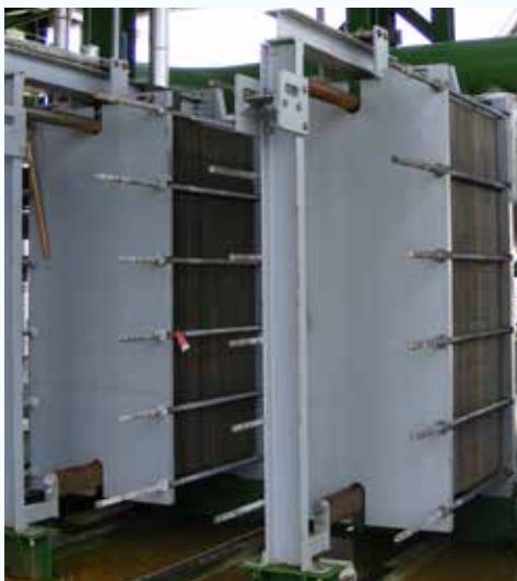
The closed loop water is re-cooled by clean cooling tower water in plate heat exchangers.
