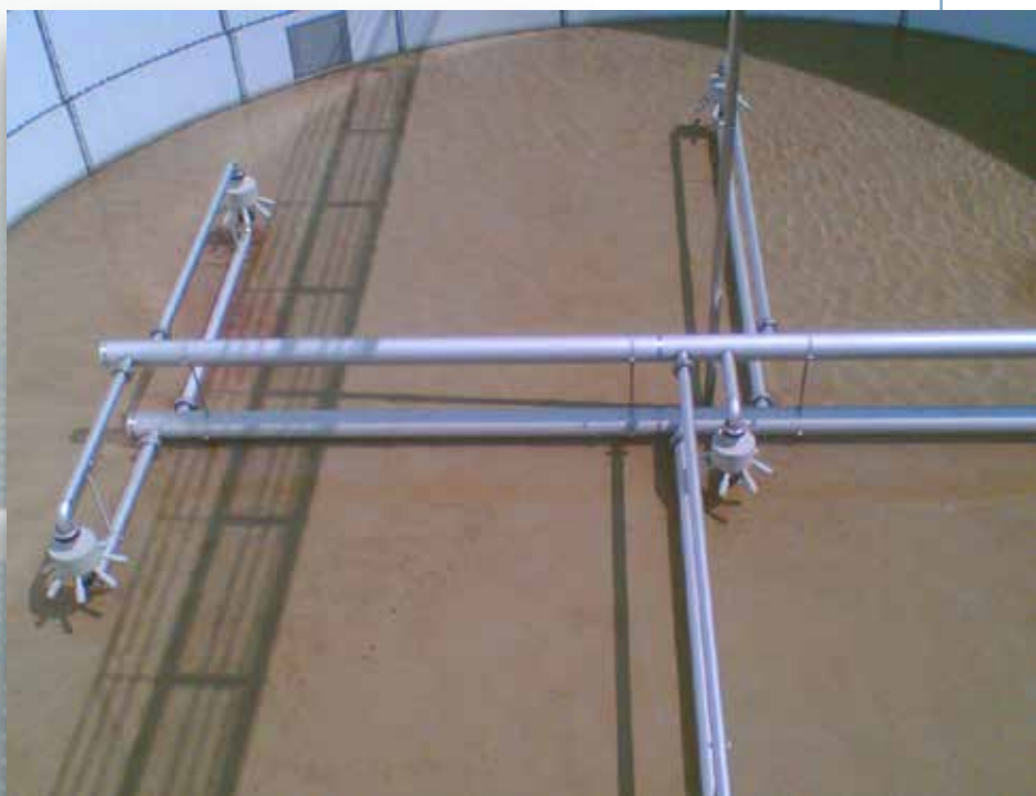
Seven-path ejectors in the 2 000 m 2 aeration tank of a laundry
