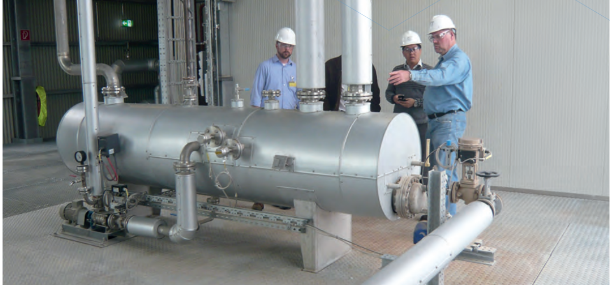
Melting vessel of a Körting ICE Condensation Vacuum System
