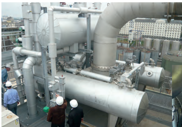
Ice condensation block completely installed at site
